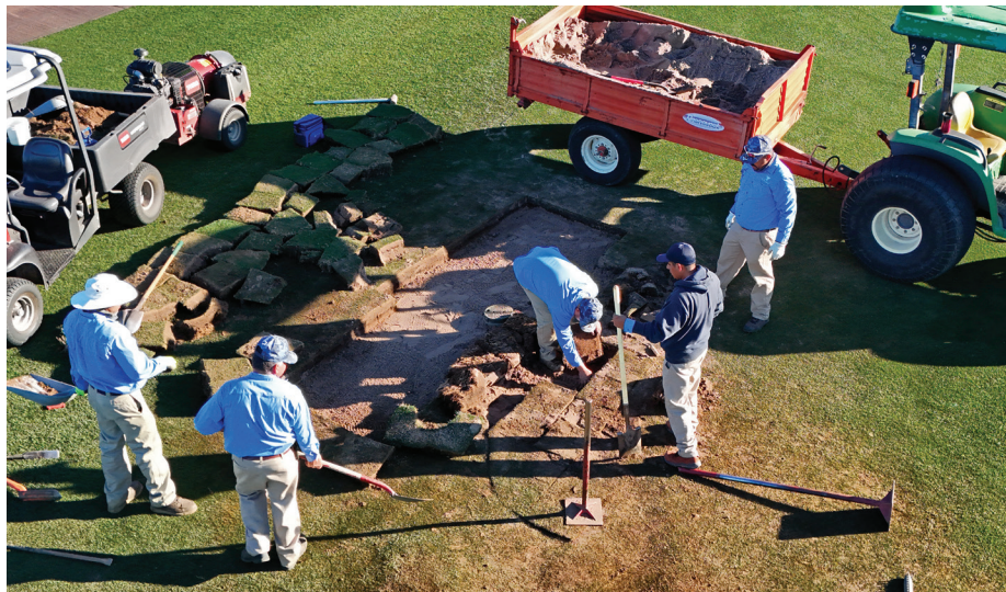
Underground leaks in lateral lines and mainlines are usually identified by wet areas at the surface. Repairs must be performed as soon as possible to ensure proper system function and minimize water waste.
