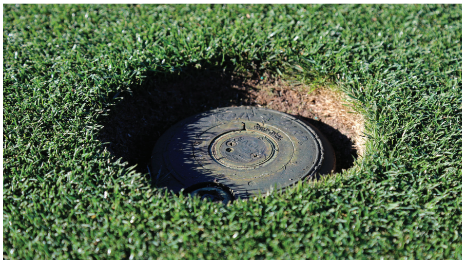
Turf growth, topdressing and sand splash from bunkers can elevate the surface around sprinkler heads. Low heads eventually need to be raised to ensure proper water distribution.
