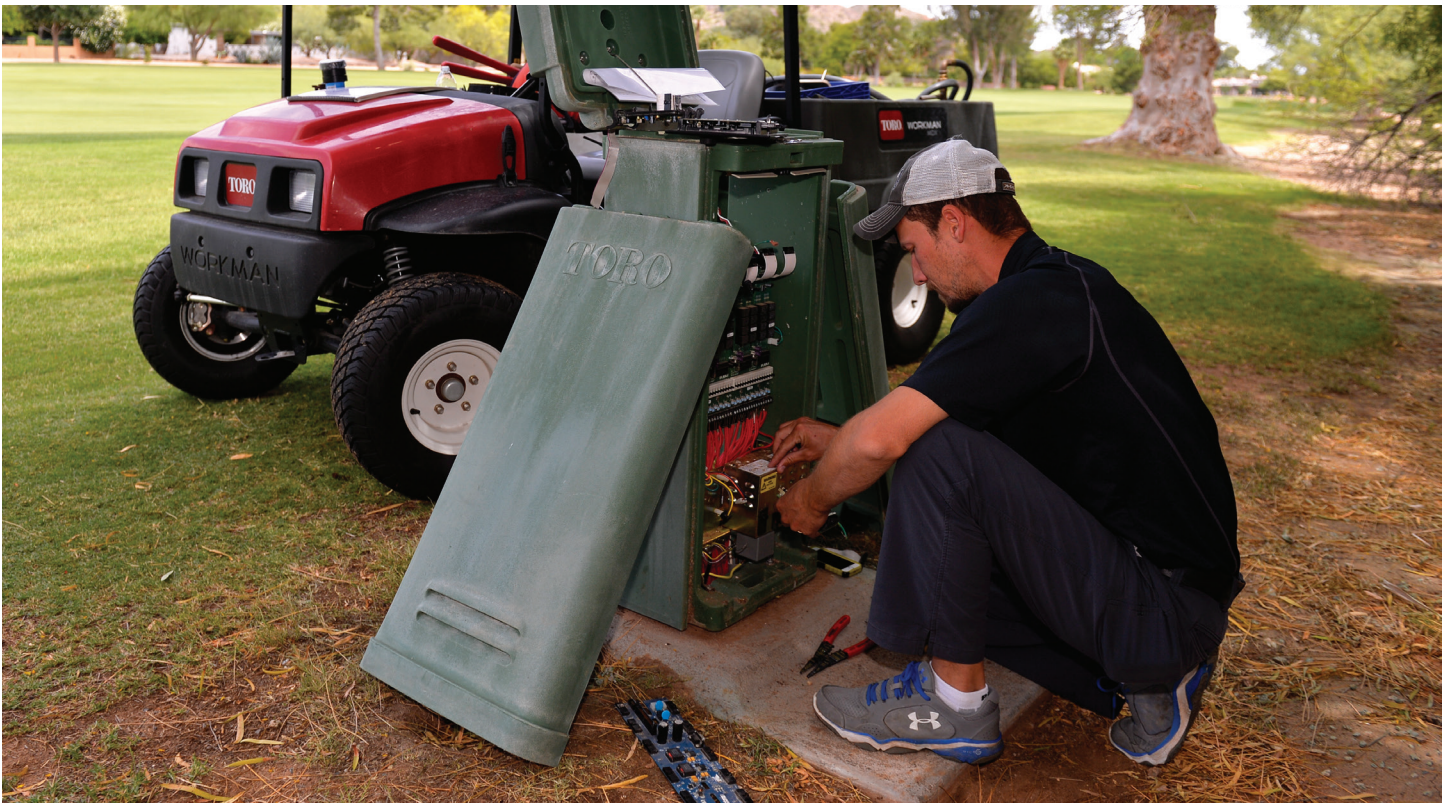
Satellites on the course should be inspected routinely for physical damage, wiring issues and the presence of pests or unwanted animals. (USGA/JD Cuban)
